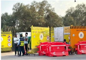
Ongoing work to cut 45,675 mangroves for the construction of the 23-km-long Versova-Bhayandar Coastal Road project. SNEHAL MUTHA
