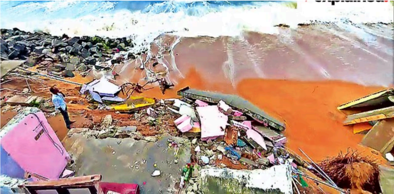
Houses damaged after water enters inside due to swell waves in Kollam, Kerala, in March. (ANI Photo)
