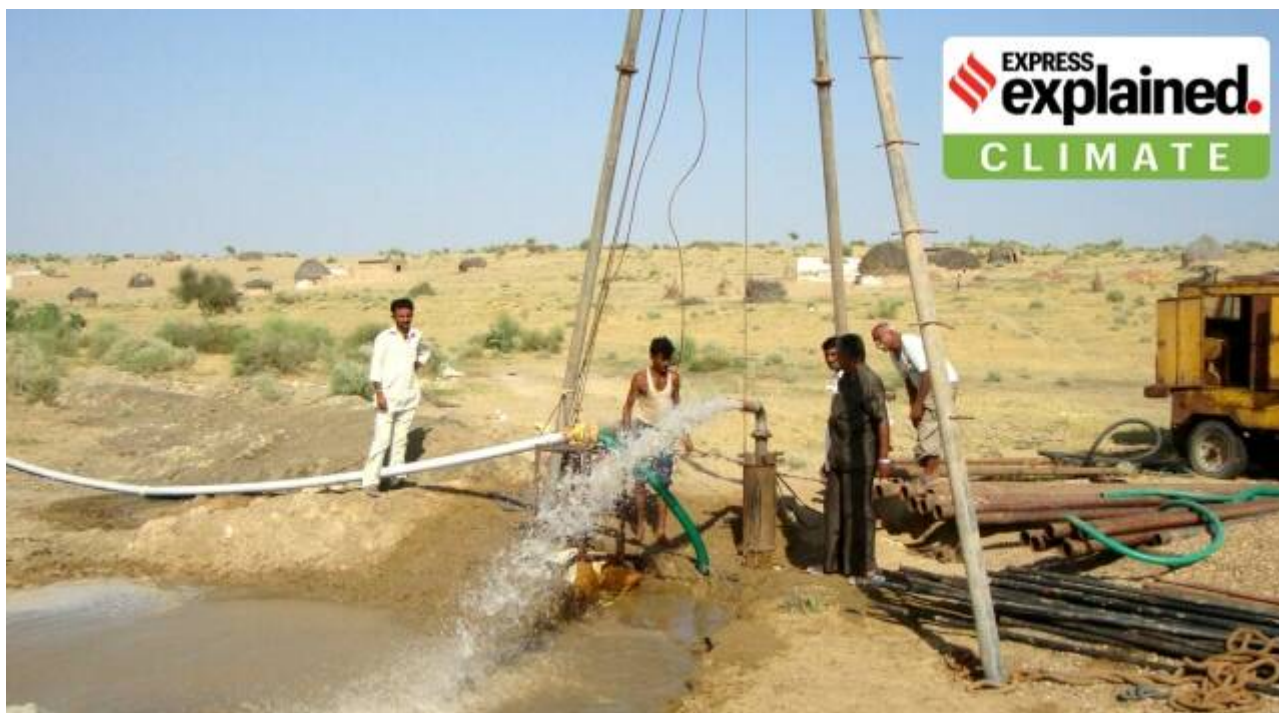
A tubewell extracting groundwater in Rajasthan. (Photo: Rohit Jain Paras/ Express Archive)
