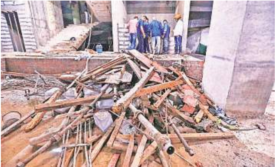
Fire officials inspect the accident site in Ahmedabad. Nirmal Harindran
