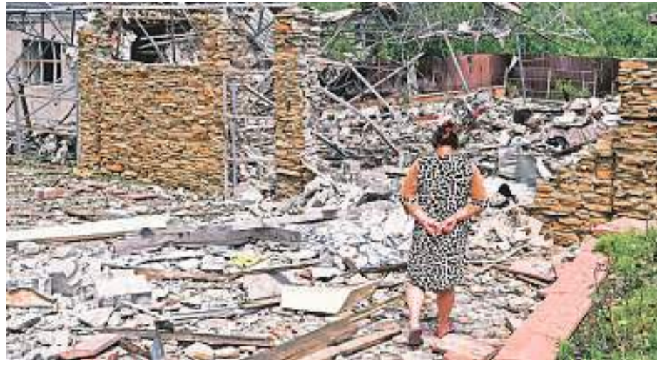
A building damaged by an overnight missile strike in Sloviansk, Ukraine, on Wednesday. AP
