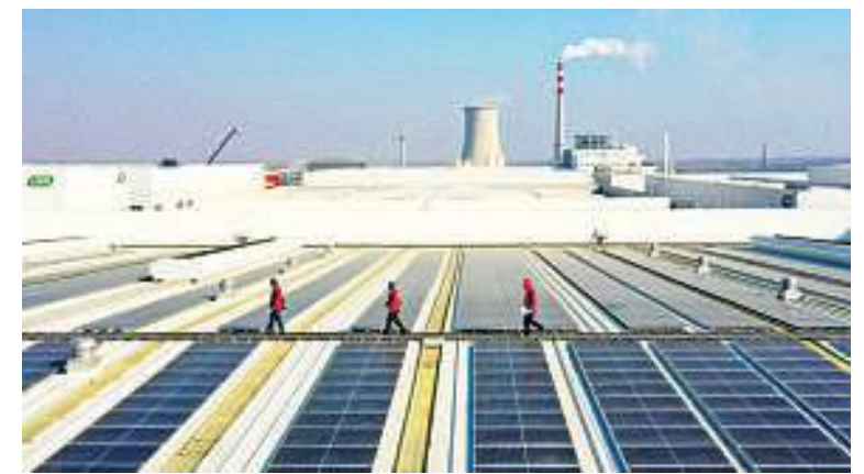
Workers carry out maintenance work on a rooftop photovoltaic power station in Mingguang, Anhui province, in December. SONG WEIXING / FOR CHINA DAILY
