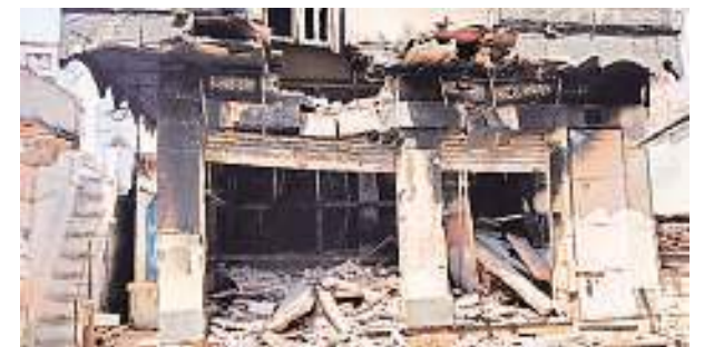
A damaged building in Karauli. Hamza Khan
