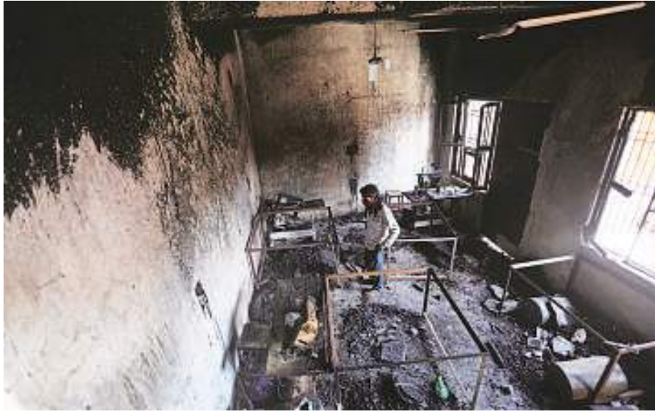
The inside of a house that was set on fire by a mob in Agra on Friday. Gajendra Yadav
