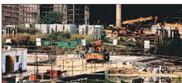
The topsoil should be stripped only up to depth of 20cm. File
