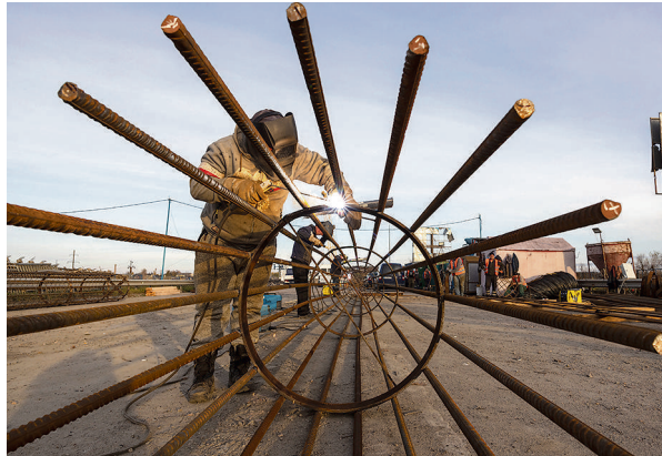
Build back: Construction under way on a bridge destroyed to block the Russian advance in Bucha, Ukraine. GETTY IMAGES
