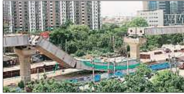
The collapse took place on the night of August 22
