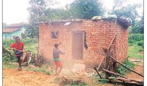
Seven houses were damaged in Kakrabela village last week
